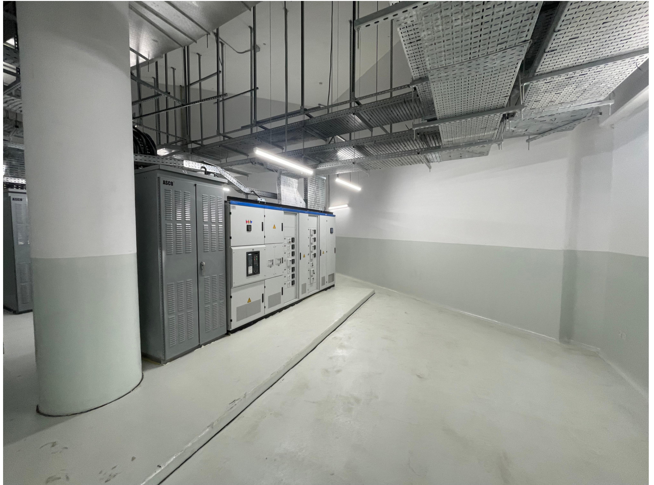
MAIN ELECTRICAL ROOM
